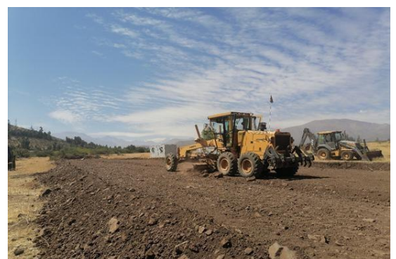
Site Grading Work on the Site of a Guadalupe Solar Power Plant in Progress, a Shot Taken on 15 March
